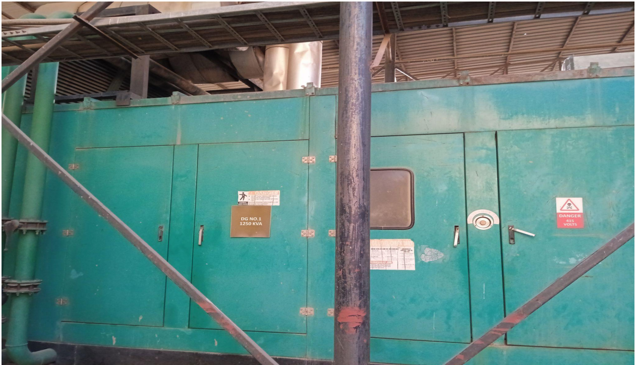
Photograph showing D.G of capacity 1250 KVA (overall 2x1250 and 1x 500 KVA)
