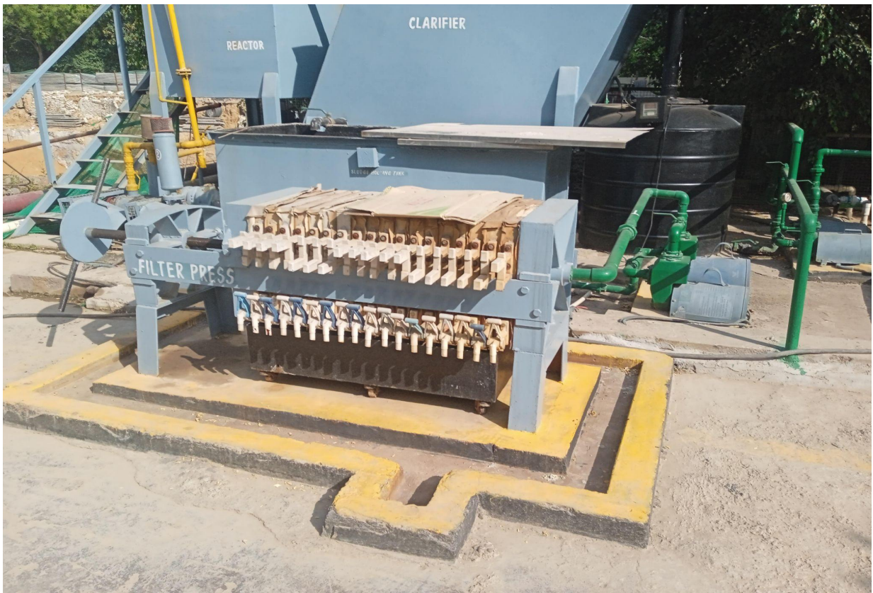
Photograph of ETP installed at the construction site
