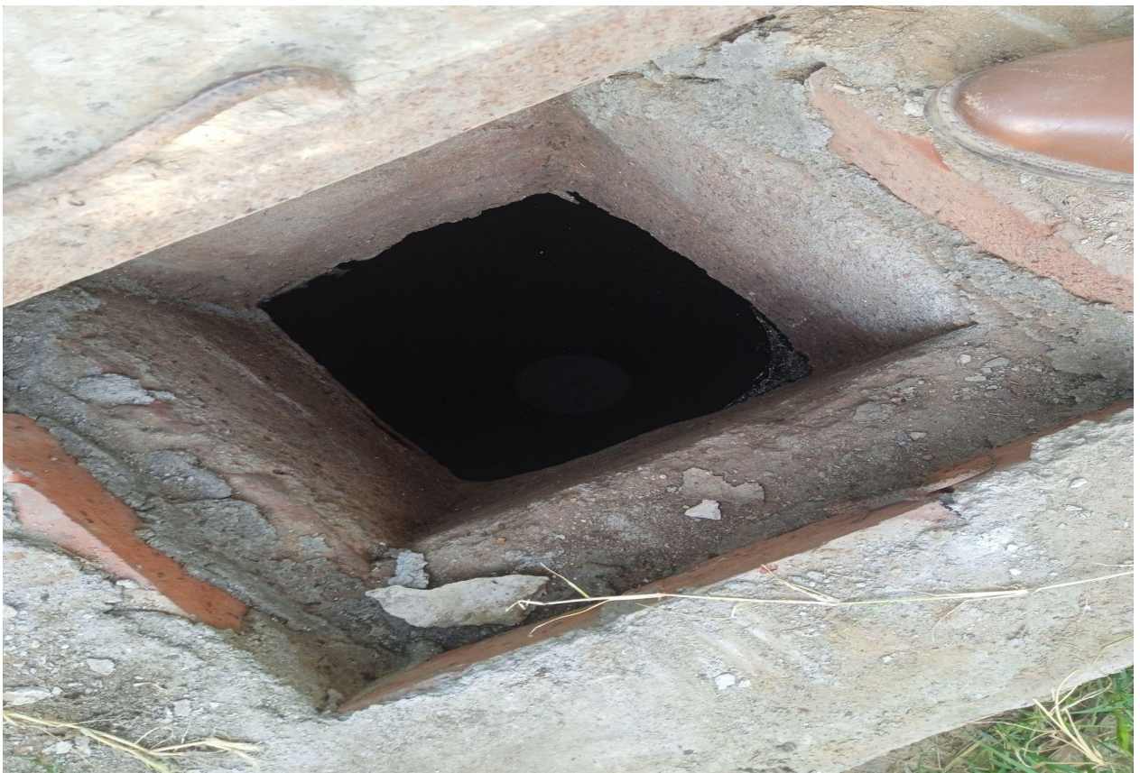
Photograph showing RWH Pit
